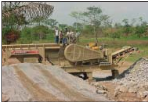
The Pioneer 3042 portable hydraulic jaw crusher and the crew in Ghana, Africa.
